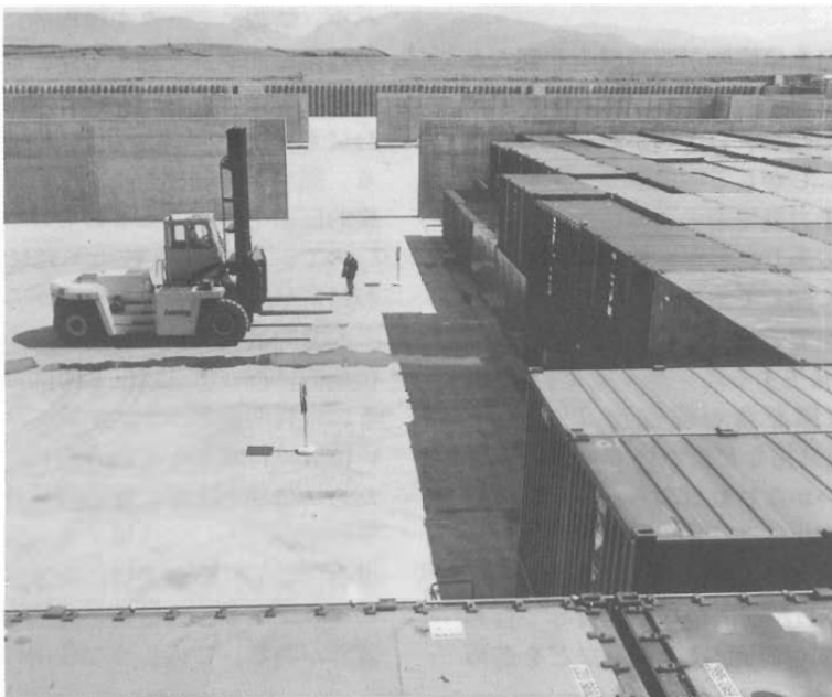
Fig.1 Engineered Concrete Vault of Low-Level Waste Disposal Site at BNF's Drigg
