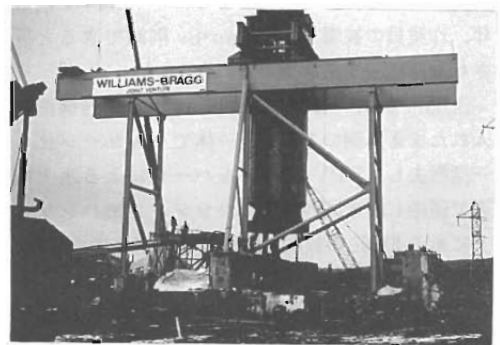
Photo 5 RPV/NST package during translation from the east bay of the lift tower to the west bay for laydown on the transporter (Ref. 291/20)
