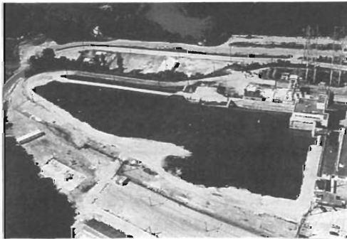
Photo 2 SSDP site status after decommissioning. Final site configuration is clearly evident. All structures to three feet below grade are removed and all voids are backfilled. (Ref. 360/18A)
