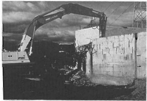
Photo 4 The pavement breaker mounted on a large hydraulic backhoe (HoeRam) in operation
